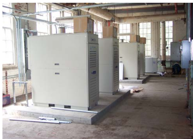
UTC PureComfort System installation at Butler Hospital
