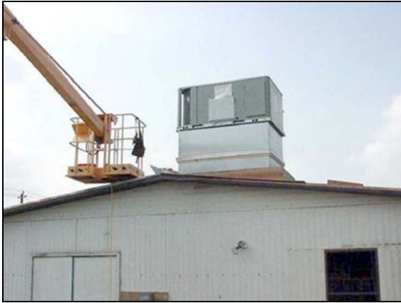
Figure 3: University of Central Florida document archive being served by Trane CDQ™ desiccant system
