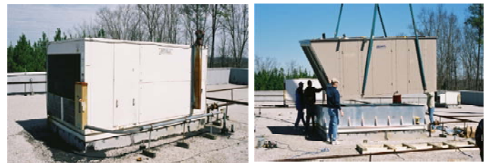
Figure 2: Old rooftop unit replaced with a SEMCO IADR on Timber Ridge School
