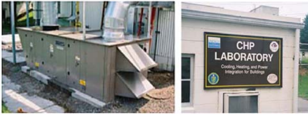
Figure 2: Photos of the IADR installed at the ORNL CHP laboratory.
