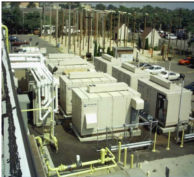
Fuel cells and absorption chillers outside Verizon central office facility
