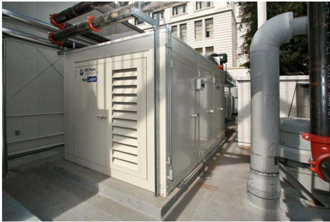
UTC PureComfort System at the Ritz Carlton Hotel
