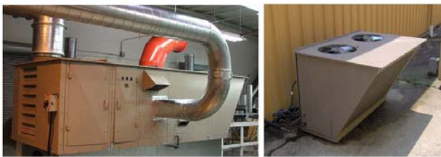
Figure 3: Photos of the IADR system installed within (main unit) and outside (condensing portion) of the SEMCO R&D Test Lab in Columbia Missouri
