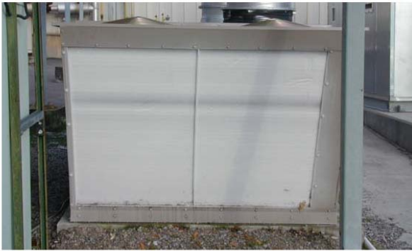
Figure 8: Photo of outdoor coil of the IADR installed at the ORNL site just before the defrost mode is initiated
