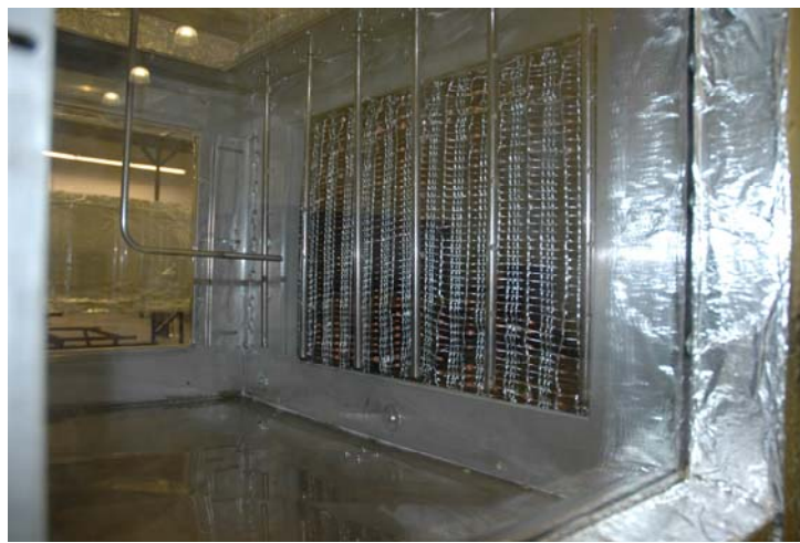
Fig. 1. Woven Graphite Fiber Heat Exchanger installed in wind tunnel.
