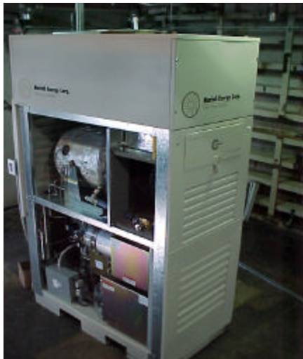
Oil Fired Mariah CHP Unit
