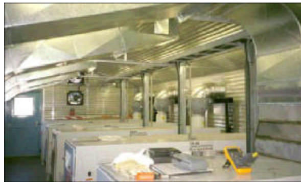
Elliott Energy Systems Installation
