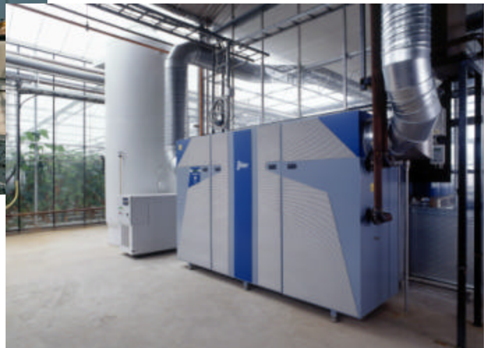
Turbec CHP Greenhouse Installation
