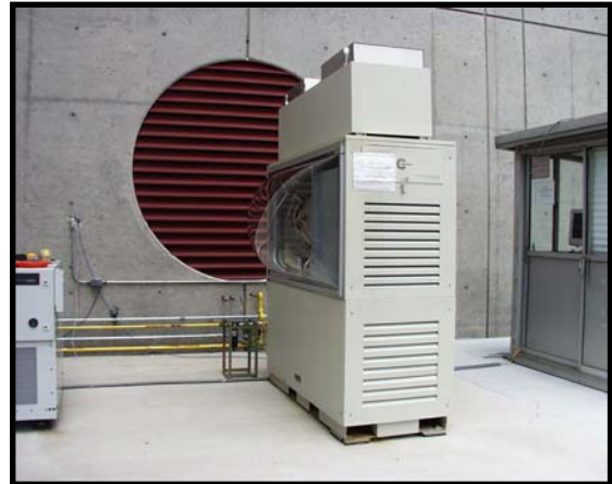
ORNL Microturbine Recuperator Test Facility
