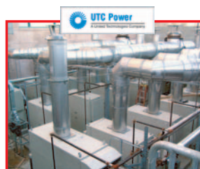
Microturbines provide ~1 MW of power.
