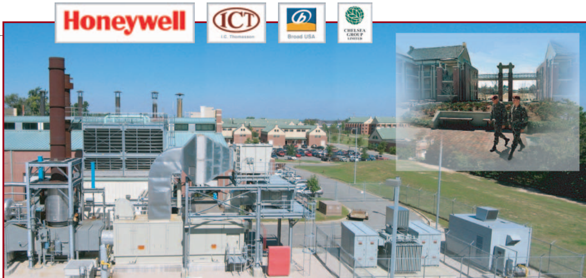
Ft. Bragg CHP plant integrates a Solar gas turbine with a Broad USA absorption chiller and a heat recovery steam generator to generate cooling and heating with no additional fuel.
