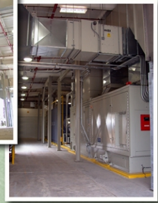
Solar gas turbine with exhaust ducted to in-line absorption chiller
