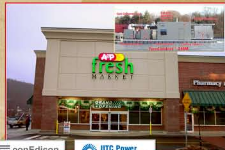
Microturbine/Chiller System in Mt. Kisco, N.Y.
