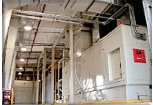
EMMC's CHP system provides power, cooling, and heating to the hospital
