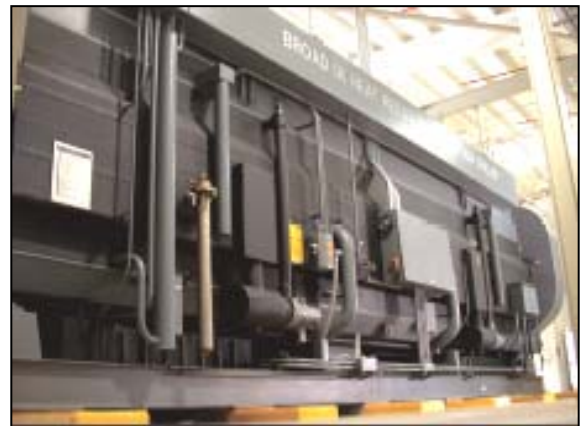
The absorption chiller produces 2,500 tons of chilled water to the District's chilled water system and turbine air-inlet cooling
