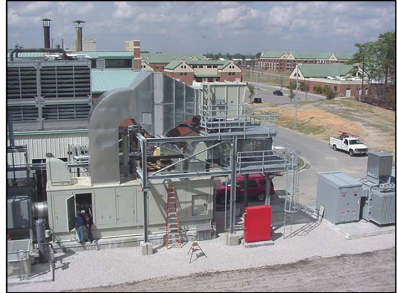
Ft. Bragg CHP plant's enclosed Solar gas turbine with exhaust ducted to in-line absorption chiller
