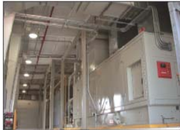
Austin Energy CHP plant's enclosed Solar gas turbine with exhaust ducted to in-line absorption chiller
