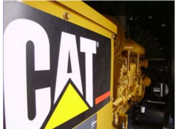
McMinnville Electric's new bio-diesel system
