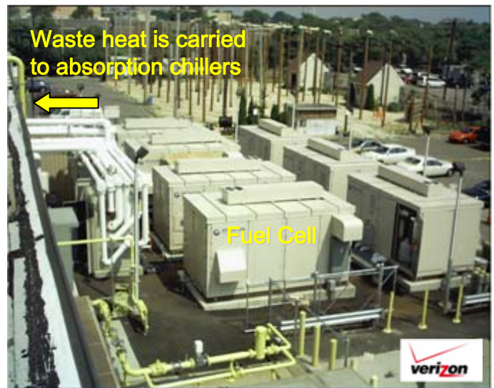
Verizon Communications, Inc. CHP System
