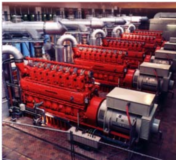
A CHP system with reciprocating engines
