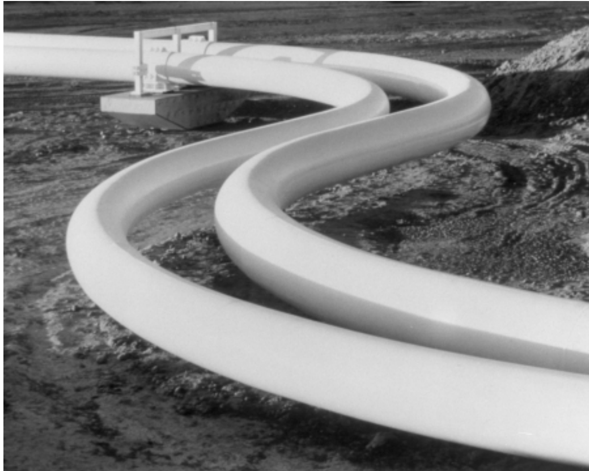
Natural gas pipeline, El Paso County, Texas. Source: U.S. Department of Energy.
