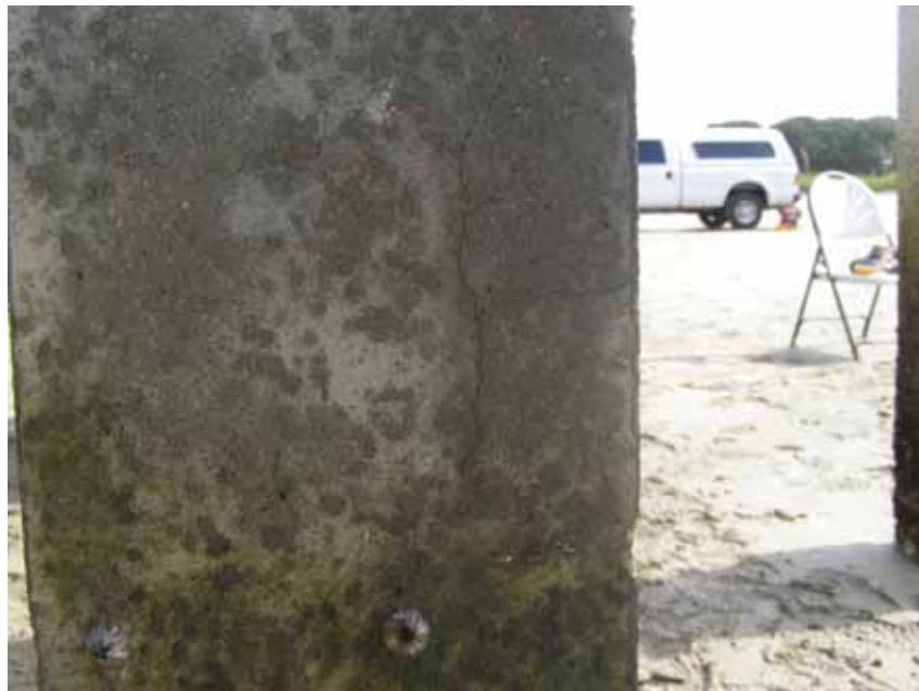
Figure 76. Photo. Cracking on a 2101 reinforced field column after 735 days of exposure.
