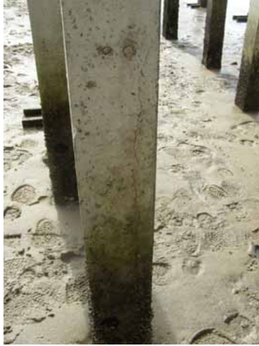
Figure 75. Photo. Cracking on a BB reinforced field column after 735 days of exposure.
