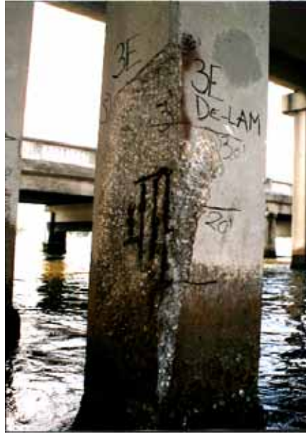
Figure 1. Photo. A cracked and spalled marine bridge piling.
