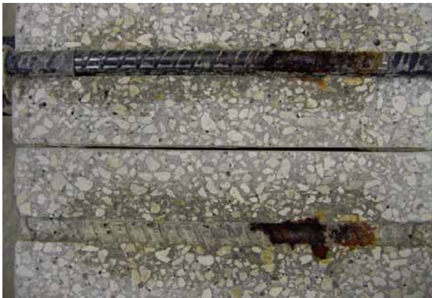
Figure 106. Photo. Top bar and bar trace for specimen MS-MMFX-2-B.
