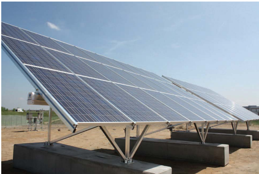
Photo from United Power's Sol Partners Installation, Colorado
