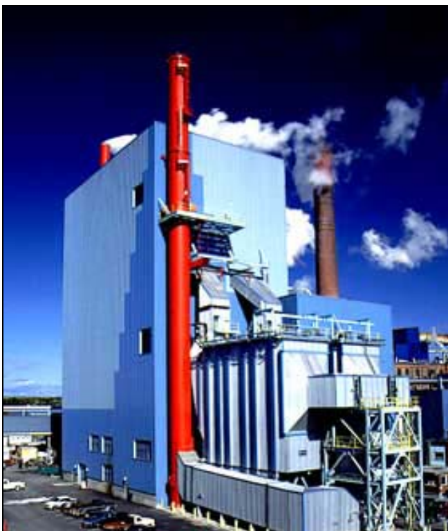
Tomlinson Recovery Boiler
