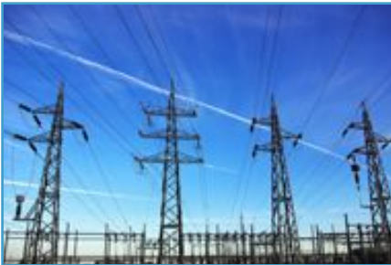
New technologies are being introduced to the electric grid.
