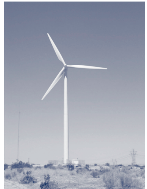
750 kilowatt wind turbine at FCI Victorville
