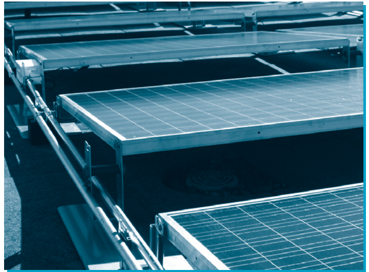
The SunRoof™ mounting system on the Dennis R. Bauer Building requires no roof penetrations or ballasting.
