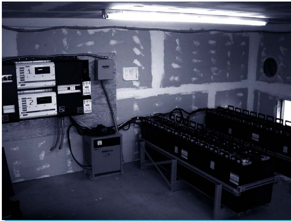
Inverter and battery system located in the generator building at Washburn Ranch, Carrizo Plain National Monument.
