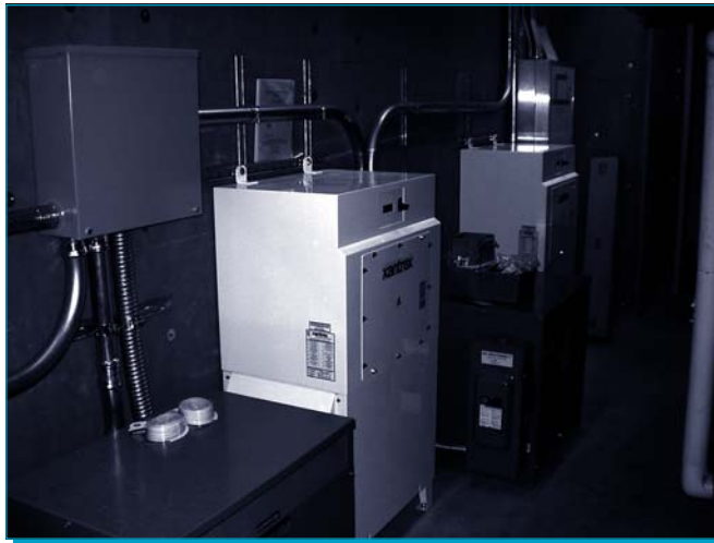
Xantrex PV-45208 inverters convert DC power to AC power.
