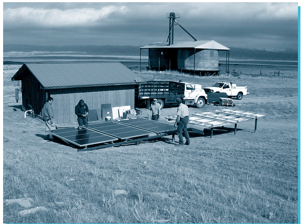
This array was installed in November 2003 by the Bureau of Land Management maintenance personnel.
