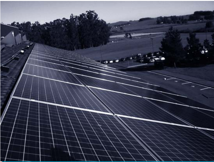
Horsley Hall Barracks' east plane PV system.
