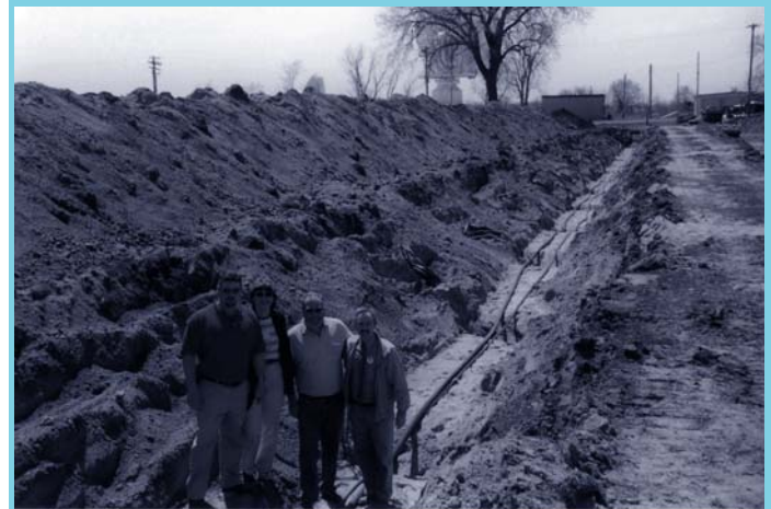
Project Partners inspect one of the trenches of the ground source loop.
