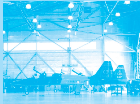
An aircraft hanger at Columbus Air Force Base with recently installed energy-efficient lighting.
