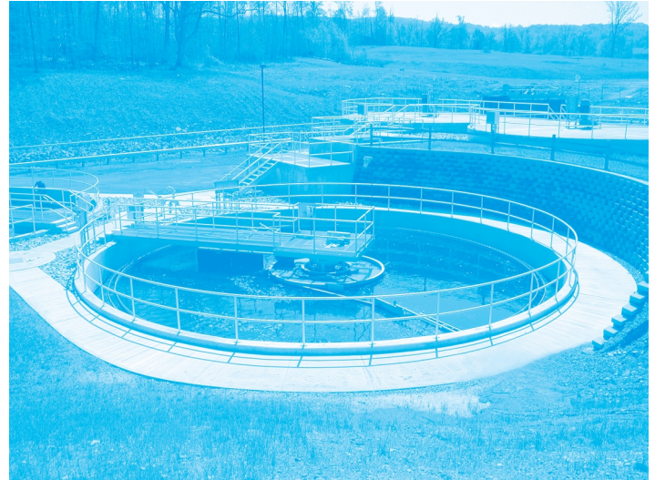
Wastewater treatment digester gas can yield methane fuel.
