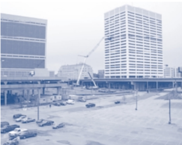
Crane replaces chillers in Richard B. Russell Building in Atlanta, Georgia, January 2000.
