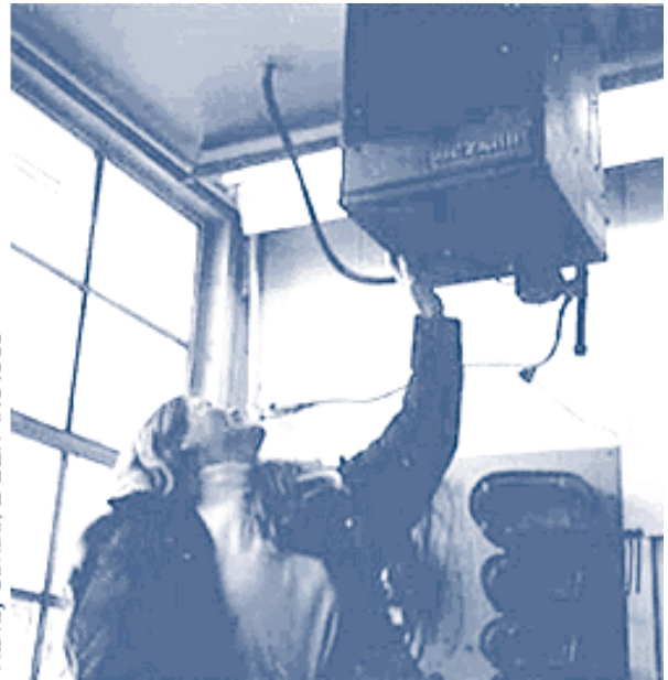
A SAVEnergy auditor inspects a unit heater at the Great Sand Dunes National Monument.
