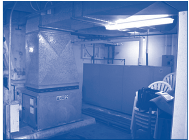
Mechanical room for Building 2000 showing Air Handling Unit on Guam Navy base
