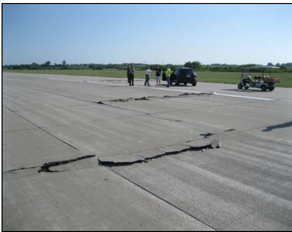
Runway Pavement Blow-up
