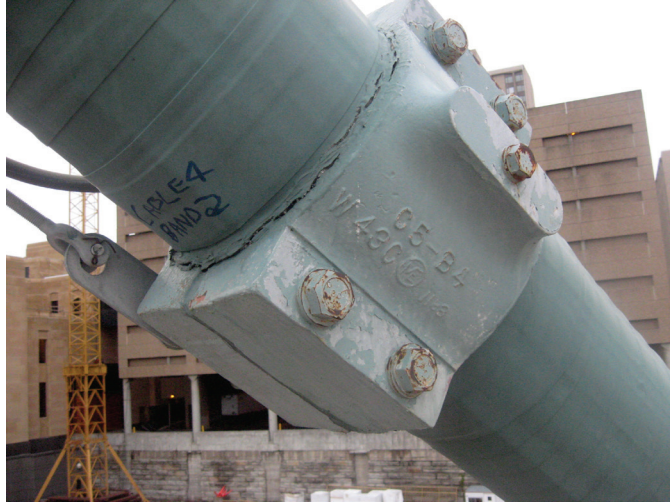
Figure 1-6 Photo showing a cable band with no suspenders
