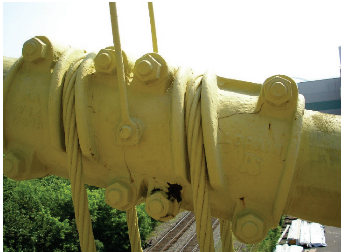
Figure 1-7 Photo showing a cable band with suspenders
