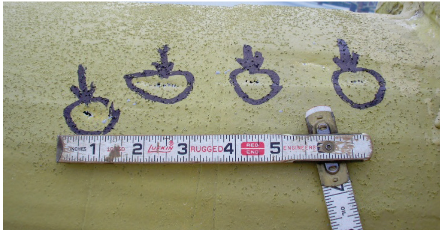
Figure 1-8 Inspection photo showing small perforations in the cable wrap which is a potential water ingress location
