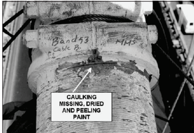
Figure 2-8 Photo showing damaged caulking and paint at a cable band (taken from NCHRP Report 534 )
