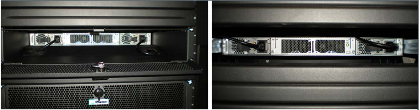
Figure 4.9. Server cowlings force air to flow through, rather than around servers. Left: server with cowling installed. Right: server without cowling installed. Photo by Michael Sheppy, NREL/PIX 19936
