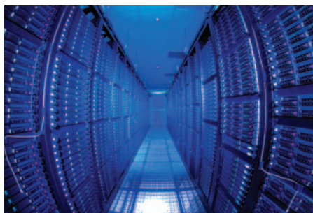
Figure 5. Grid Computing Center interior. Photo courtesy of FNAL
