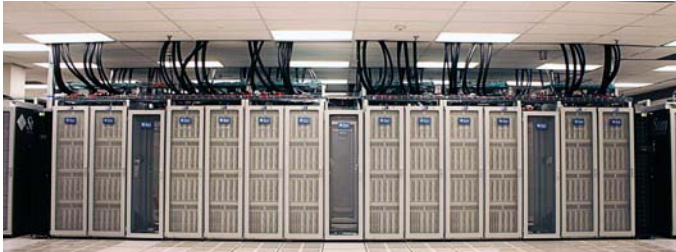
Figure 3. Sandia Labs' HPC clusters. Photo courtesy of Sandia National Laboratories
