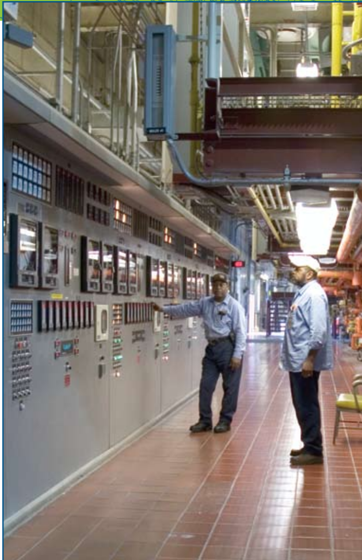
Over the past 10 years, the National Institutes of Health has taken steps to reduce its energy use through gradual improvements to the Bethesda Campus Central Utility Plant. Projects have included replacing old, inefficient chillers with ultra-efficient, large capacity chillers; retrofitting oil-burning boilers to use natural gas as the primary fuel; replacing the utility distribution system with larger capacity lines to reduce heat-loss and chilled water operating pressures; and installing a 23 megawatt cogeneration unit that is 85 percent efficient. These measures have resulted in savings of nearly 10 million kilowatt-hours, 24 million gallons of water, and $1 million in annual energy costs.
