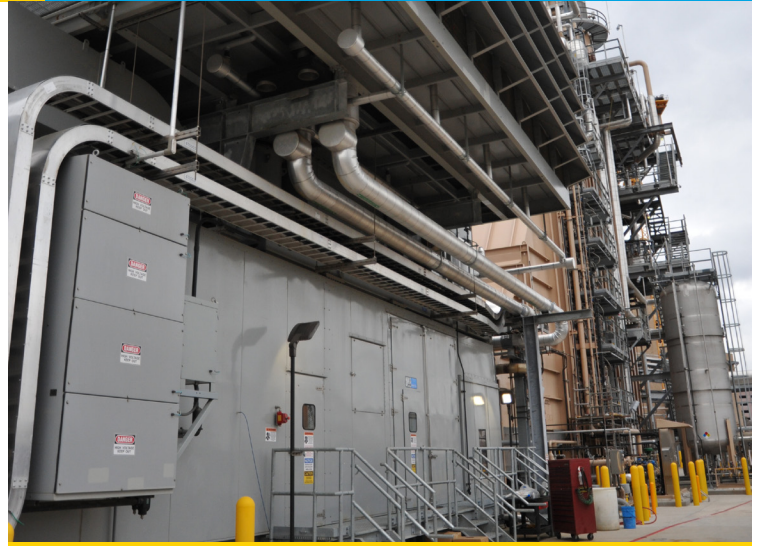
The CHP System at the Texas Medical Center. Photo courtesy of Thermal Energy Corporation
