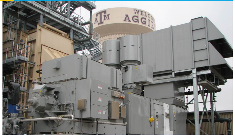
The CHP System at Texas A&M University. Photo courtesy of Texas A&M University
