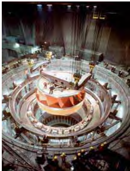
Photo: Third Powerhouse turbine runner being installed in 1974. Turbines are 16'8" in diameter, weigh approximately 1 million pounds each, and produce up to 805 megawatts of power.
