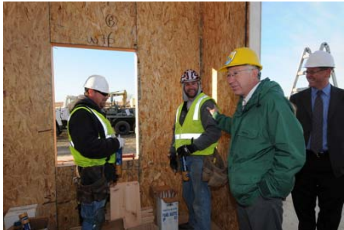
Interior Secretary Salazar tours the headquarters/visitor contact building under construction at the Audubon NWR in North Dakota. The project was funded by ARRA.
