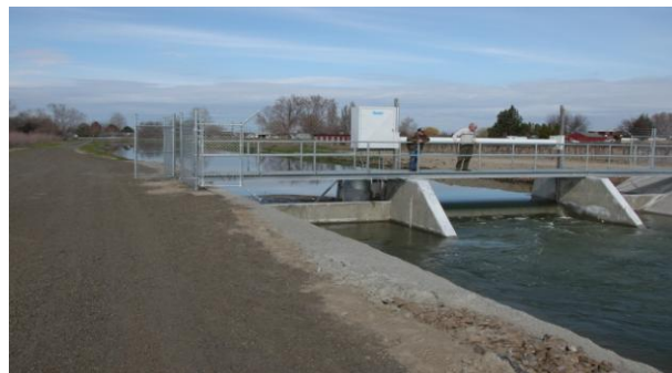
Figure 2. New automated check controlled from SVID office, reduces operational spills and can be adjusted remotely.
