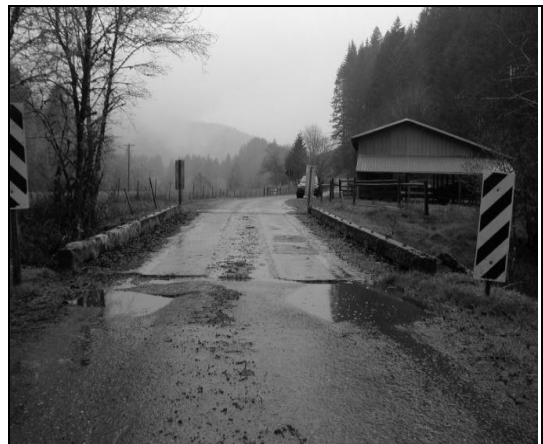
Bridge approach work is a typical ongoing maintenance need for Western Oregon roadways. Ditch clearing needs and culvert replacements are also in constant demand.
