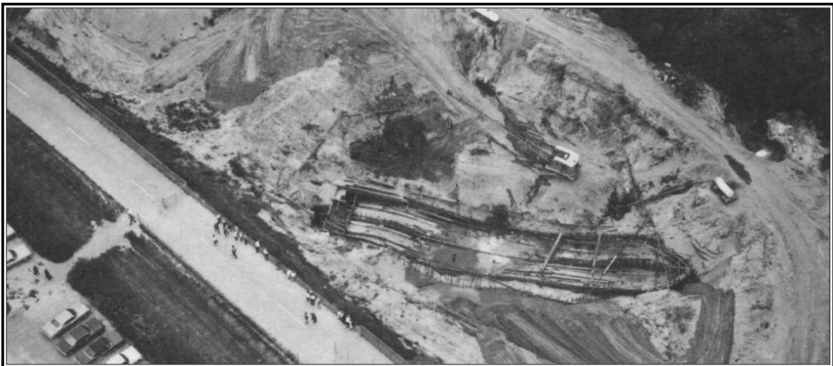
Figure 56. Aerial view of the steamboat Bertrand excavation, Missouri River, Nebraska, 1969. (National Park Service)
