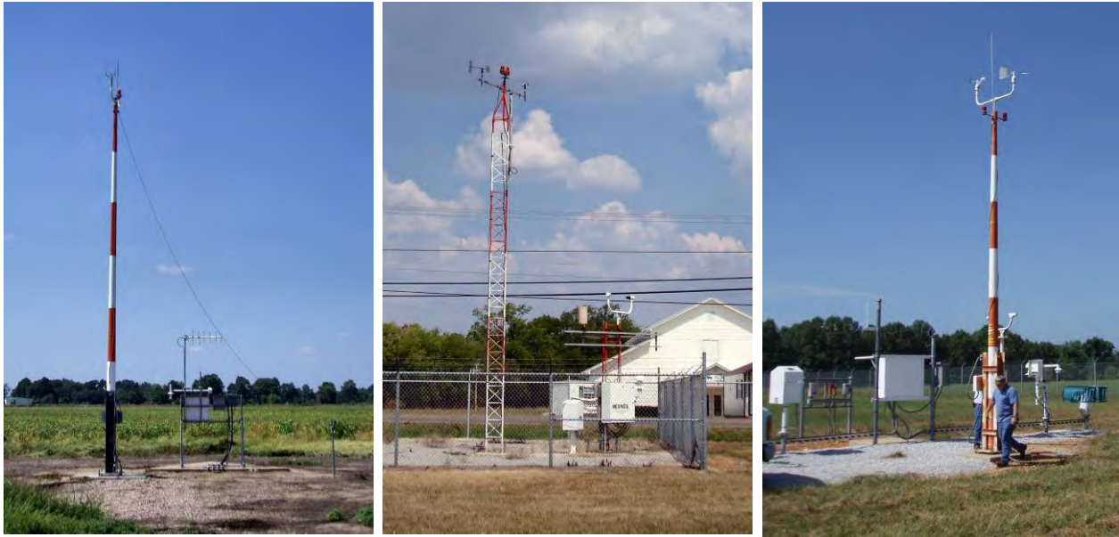
Figure 2-10. SAWS, AWOS and ASOS Station Installations.
