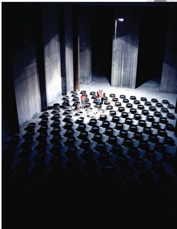
The canister storage building vault where workers are seen moving a tube to the lift site with special wheeled dollies.
