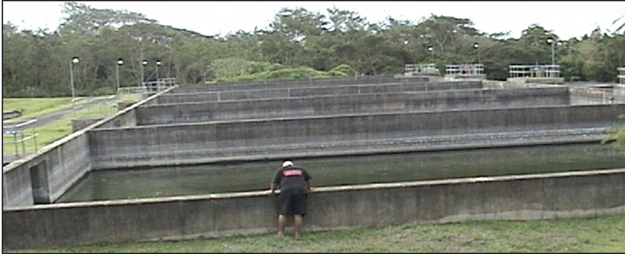
Samoa's water filtration system in Vailima, Upolu. Vice Chairman Tuaoalo examines the structure.
