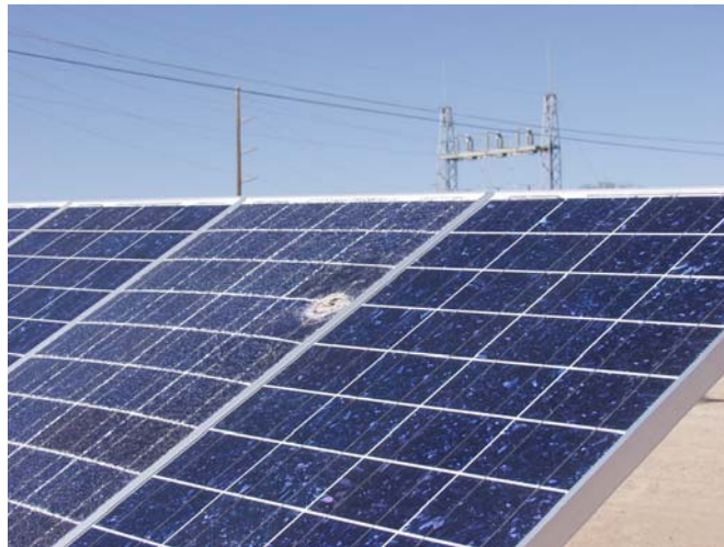
Figure 7: Vandalized NTUA PV Module
