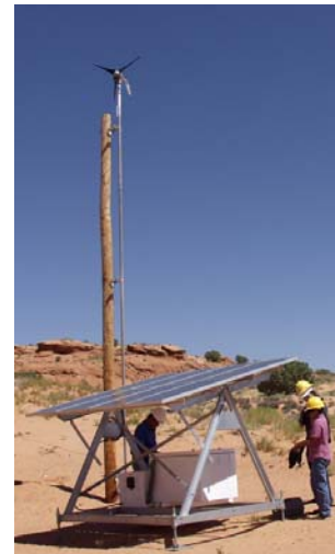
Figure 7. Phase I Small wind turbine mounted on a utility pole.
