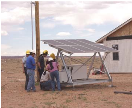
Figure 8. The Phase II 880 Watt small wind hybrid unit.
