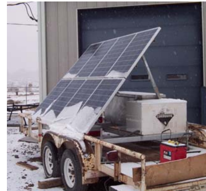
Figure 4. Integrated 660 Watt unit ready to be deployed on NTUA trailer.
