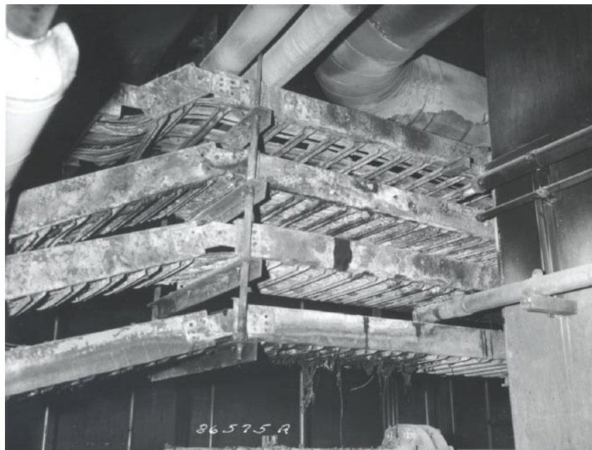
Figure 2 Browns Ferry cable trays after the fire, showing damaged cables
