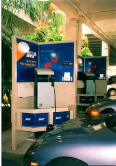
Figure 5-11. Level 2 public charge station in a mall parking structure with lighting, access control system, and a customer service speaker phone
