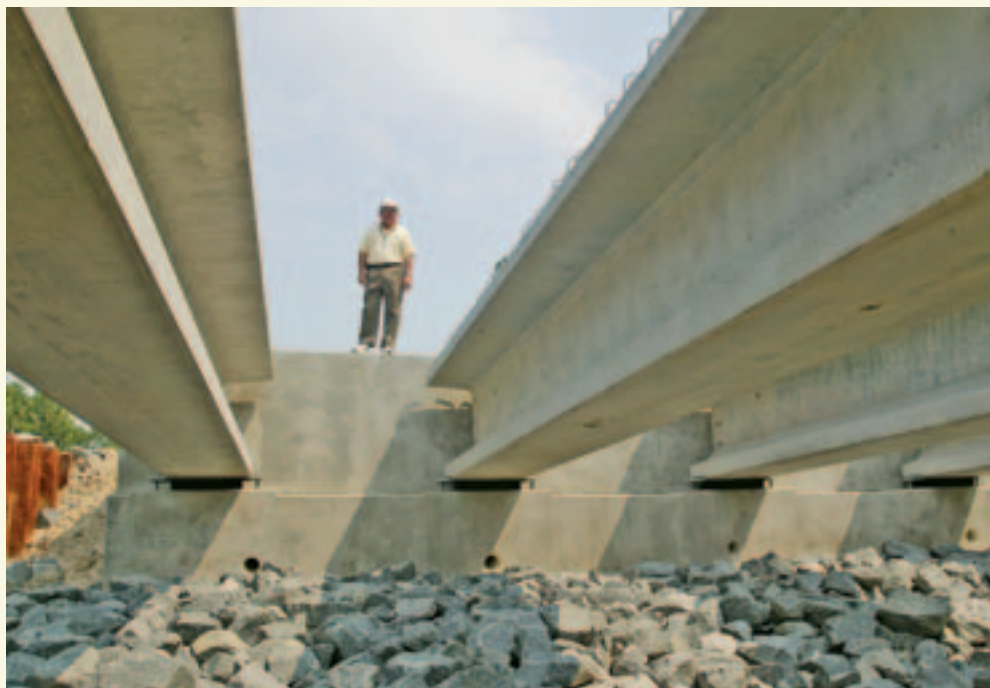
Route 17 Project Manager Wayne Williams with the Virginia Department of Transportation looks at a new pair of parallel bridges. Animals can cross under the bridge on the rocks. There will also be a natural wildlife walkway installed underneath the bridge. (Tom Saunders/Virginia Department of Transportation)
