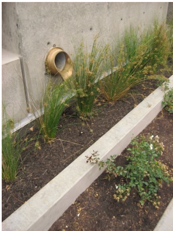
Figure 9. Disconnected downspout discharging to planter box.
