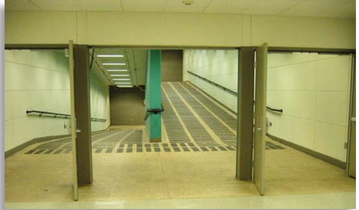
This ramp is part of a means of egress system. Photo courtesy Keith Heckler, Rockville Fire Department, Maryland.
