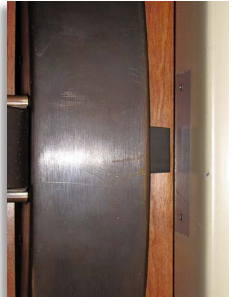
The strike plate is missing from this exit hardware device, compromising its ability to hold the door closed.
