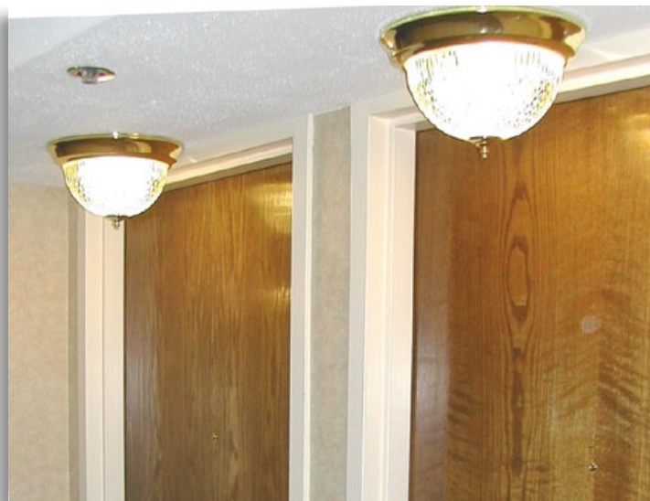
These luminaires might create a bumping hazard for a tall occupant.
