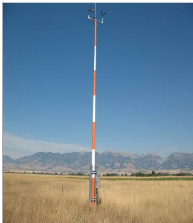
Figure 6-35. Weather Equipment Sensor Pole
