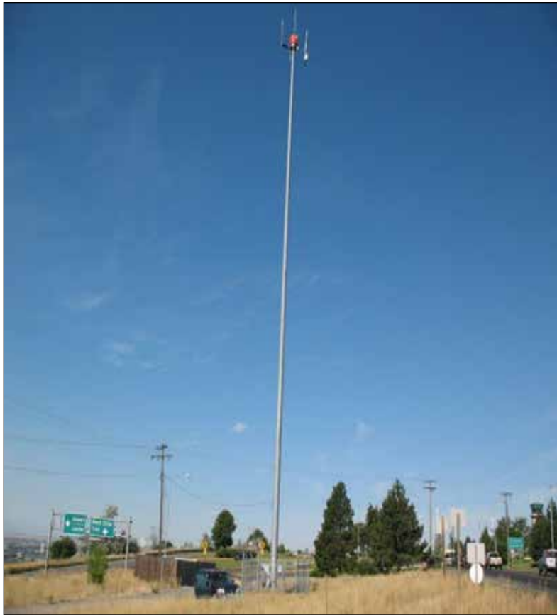
Figure 6-36. LLWAS Sensor Pole
