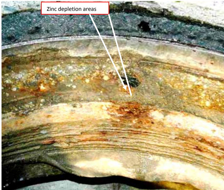
Figure 13. A36 Galvanized Light Base - Aluminum Light Fixture Removed
