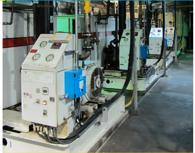
Verso Paper Corp. is improving energy efficiency at paper mills with heat recovery and automatic load controls for multiple air compressors.
